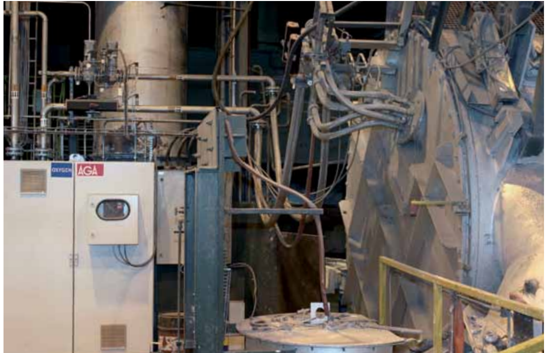
The alloying and casting furnace at Stena Aluminum was converted to Low-temperature Oxyfuel in 2009.
